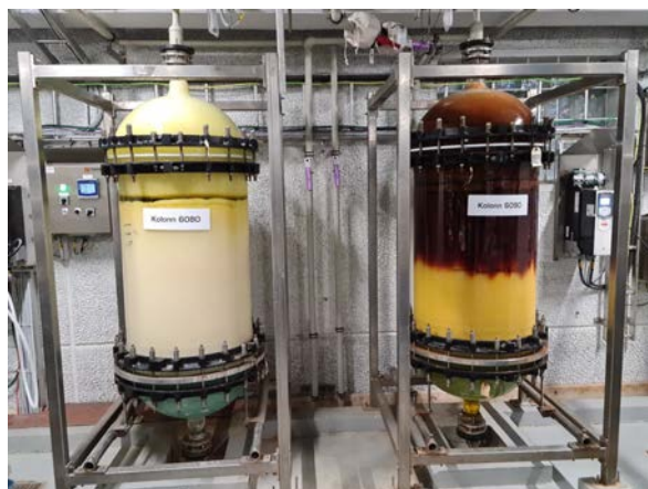
Left: Column packed with SuperLig® 2
