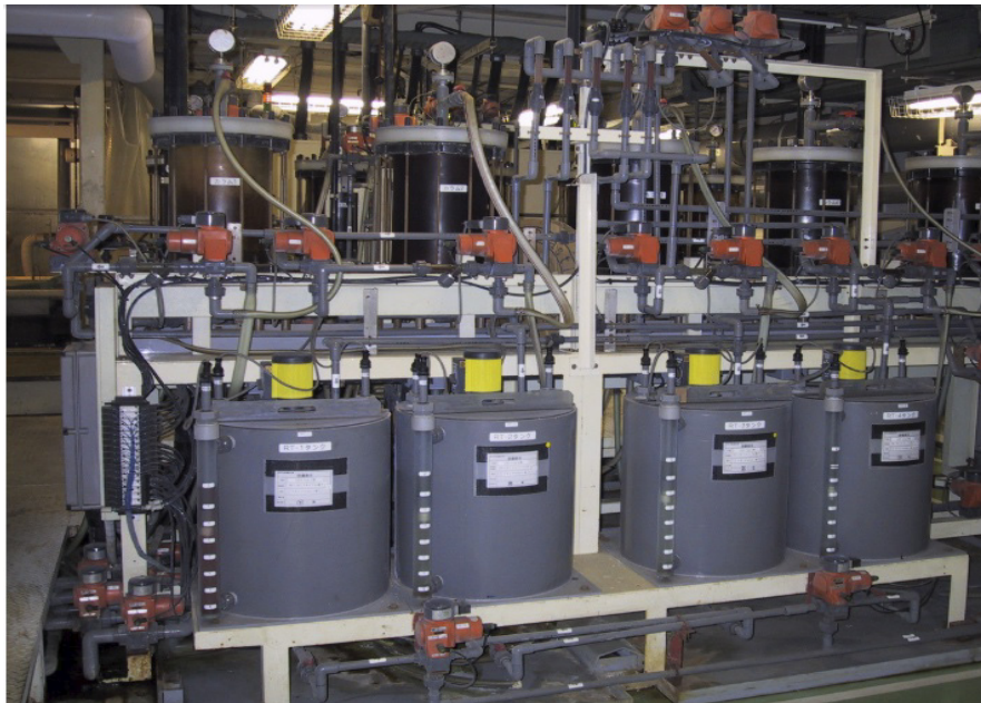
Figure 3. MRT Rh refining system at Tanaka Kikinzoku Kogyo K.K. [39,52a].
